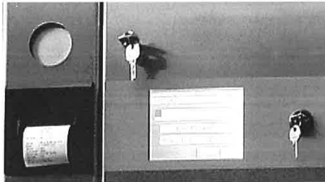
Figure 4-4: Operating end control panel
